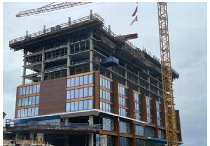
Fig. 8: The Snoqualmie Casino Hotel structure is a reinforced concrete frame with post-tensioned slabs and two shear wall cores. The layout was designed to accommodate a column-hung forming system for slab construction, thus eliminating the need for shoring and reshoring and facilitating early access by MEP and finish workers
